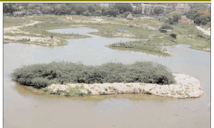
The Ecological restoration work in progress at the Adyar estuary in Chennai.
